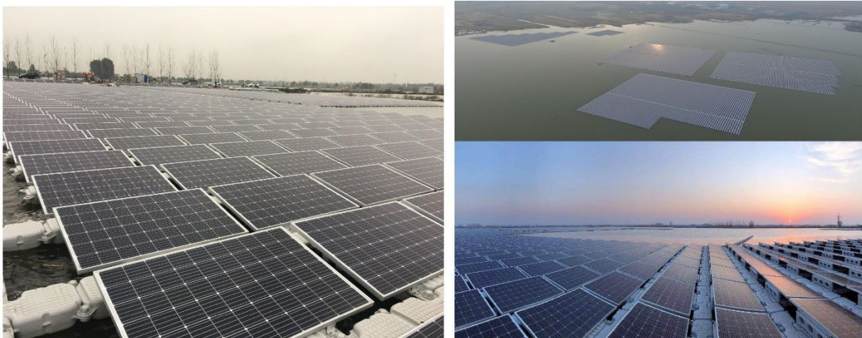
Fig. 4 HDPE technology based floating solar panels
